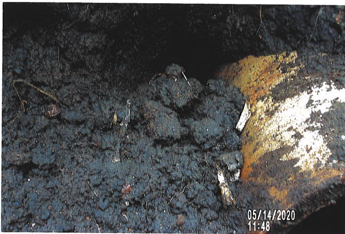
PICTURE # 3544 IS LOOKING SW ON EAST SIDE OF TILE AT 5.5' LONG SOIL ERODED CAVITY IN BLOWOUT # 28 FROM GPS # 118
